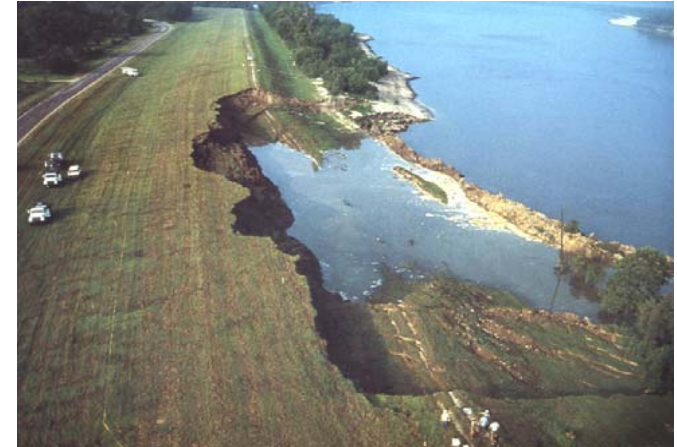
Picture of levee breach
