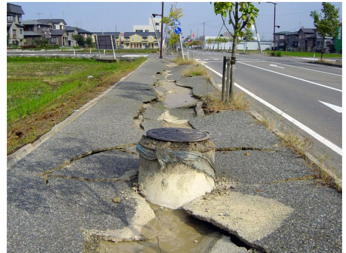
Liquefaction from 2004 Chuetsu earthquake
